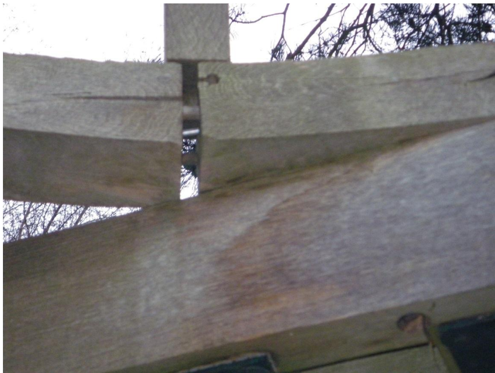
Section 1: showing opening of joints in the timber superstructure
