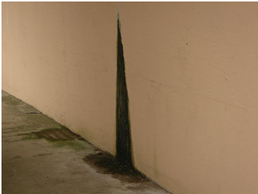
Section 2: water seepage through the retaining wall.
