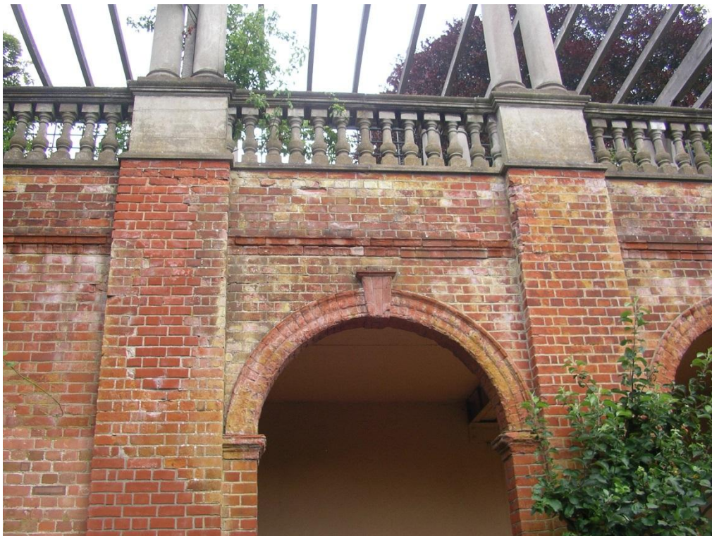
Section 1: Brickwork arcade to lower level walkway showing deterioration due to dampness.
