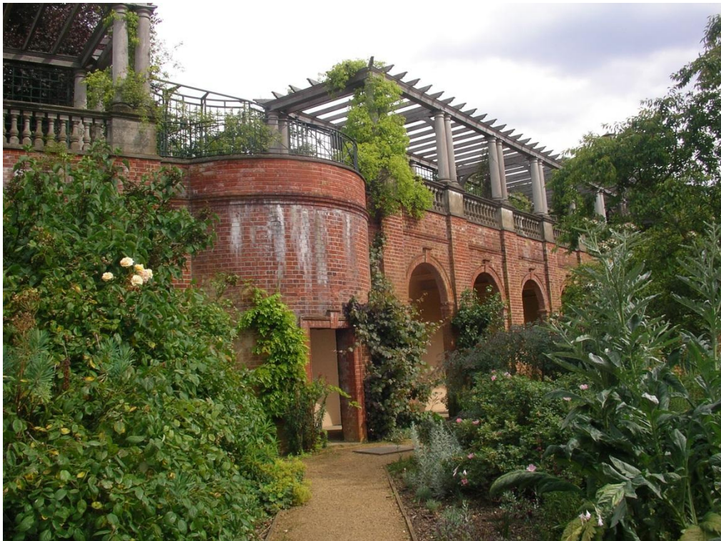
Section 1: The rotunda feature showing unsightly efflorescence.
