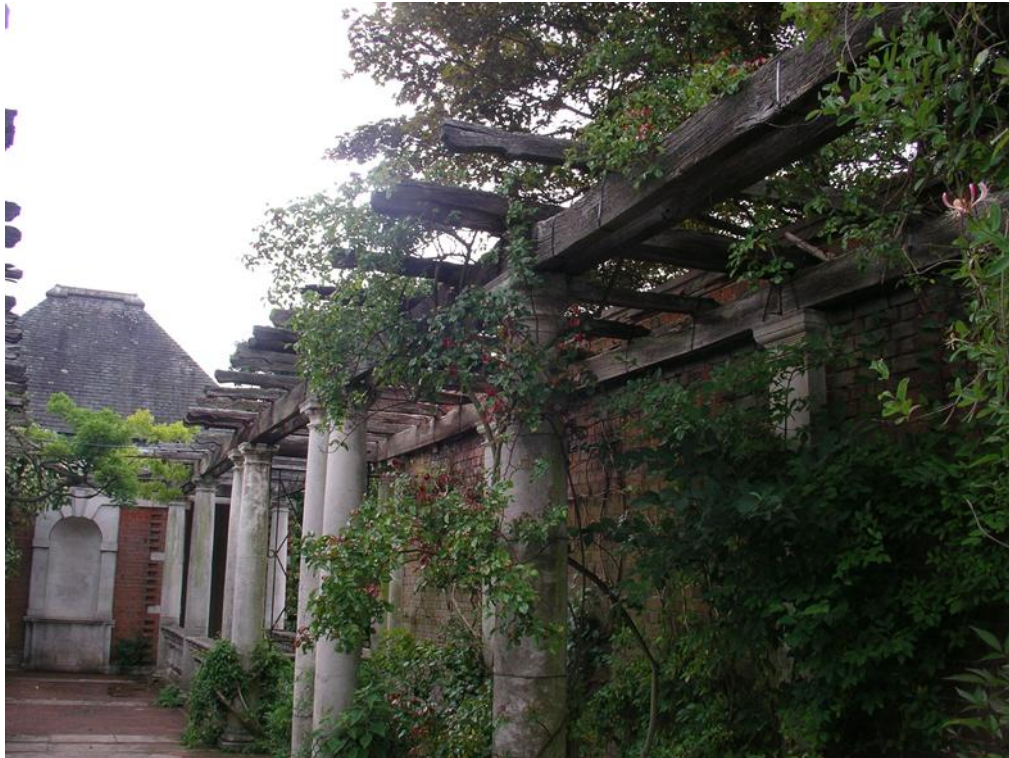
Section 2: showing timber superstructure with decayed and missing sections.
