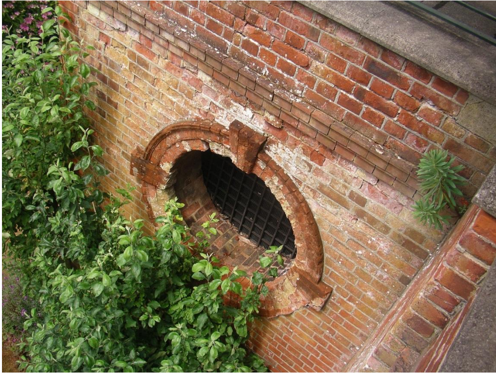
Section 1: brickwork deterioration around a circular window feature and efflorescence below the level of the structural slab to the walkway.
