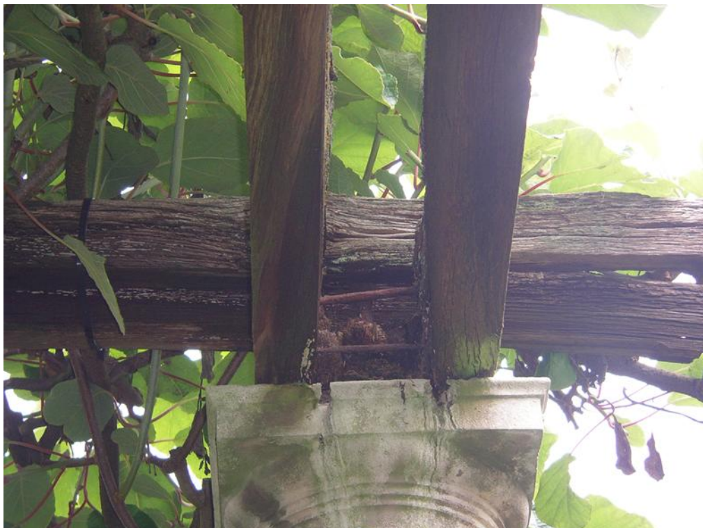
Section 2: showing decayed timbers and acid attack to Portland stone column from oak timbers.
