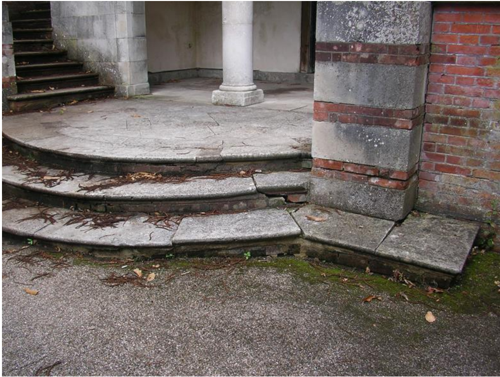
Section 2: cracked staircase at the Belvedere structure which will be repaired as part of the 2015/16 cyclical maintenance programme.
